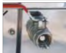
Ball valve drain
